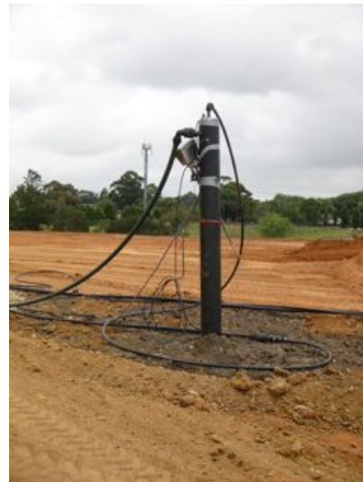
Cranbourne (VIC) - Methane extraction
